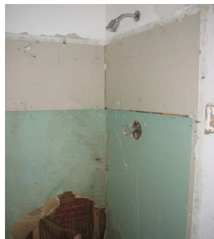
Incorrect use in a wet area
